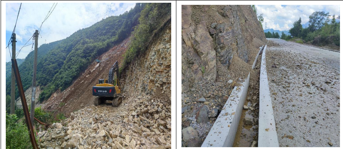
K6+660~K7+080 段边坡坍塌
